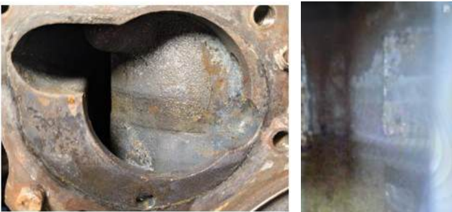
Left: Behind water pump looking at cylinder 1 casing. Right: Using a bore camera looking inside the block at the casings for cylinders 2, 3, & 4; nicely improved
